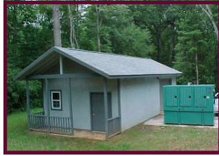
Sewer Pump Station
